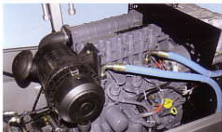
Engine compartment, right-side view
